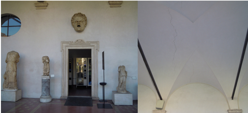
Figure 21. Wall and vault of the Cloister chosen for the humidity and lesion monitoring; the areas chosen for monitoring are shown in red.
