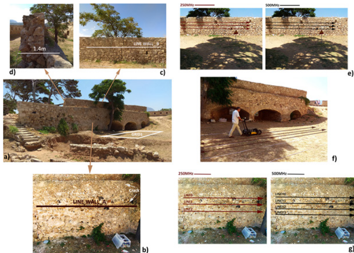
Figure 9. Details of the survey area of St Lucas Bastion: a) location of the survey grid named as GRID1, b) scan line at the front wall labelled as WALL A, c) scan line at the back of the wall, labelled as WALL B, d) the width of both walls is presented; e) orientation of the collected scans at WALL B with both antennas; f) orientation of the collected lines at the survey grid and g) orientation of the collected lines at WALL A.
