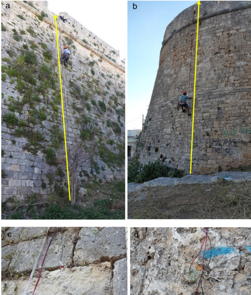
Figure 5. Layout of the vertical ERT line along the walls of the St Paul (a) and St Lucas (b) Bastions. Details of the connection between the metal nail and the wire output of the custom made multimode cable (c). Covering the metal nail with wet bentonite to decrease the contact resistance (d). Arrows indicate the direction of the ERT profiles.
